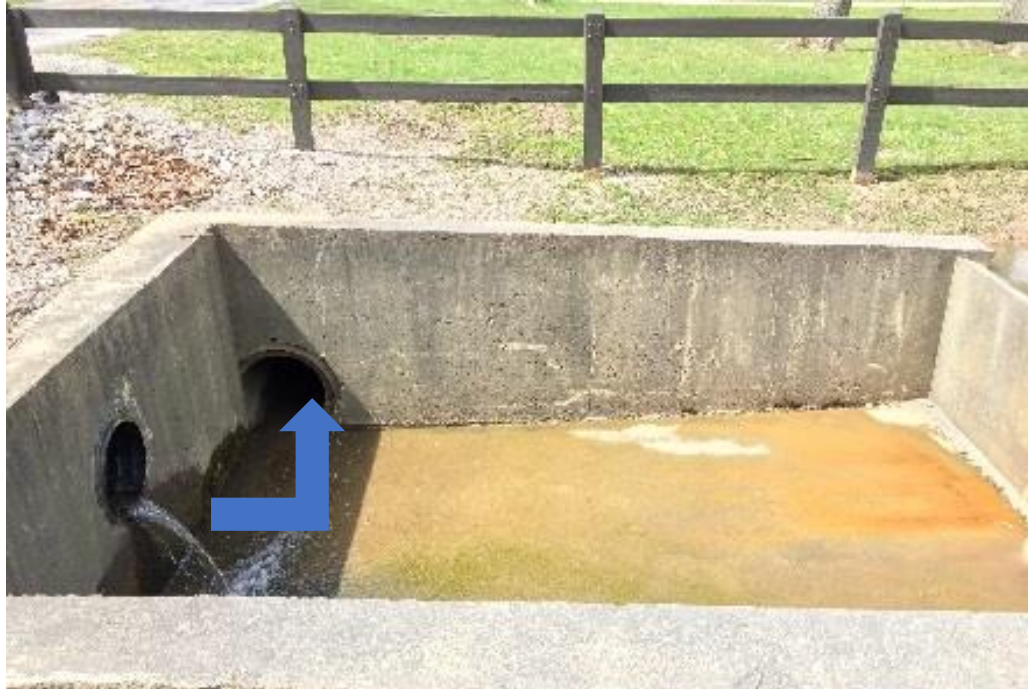
Poorly designed box culvert
