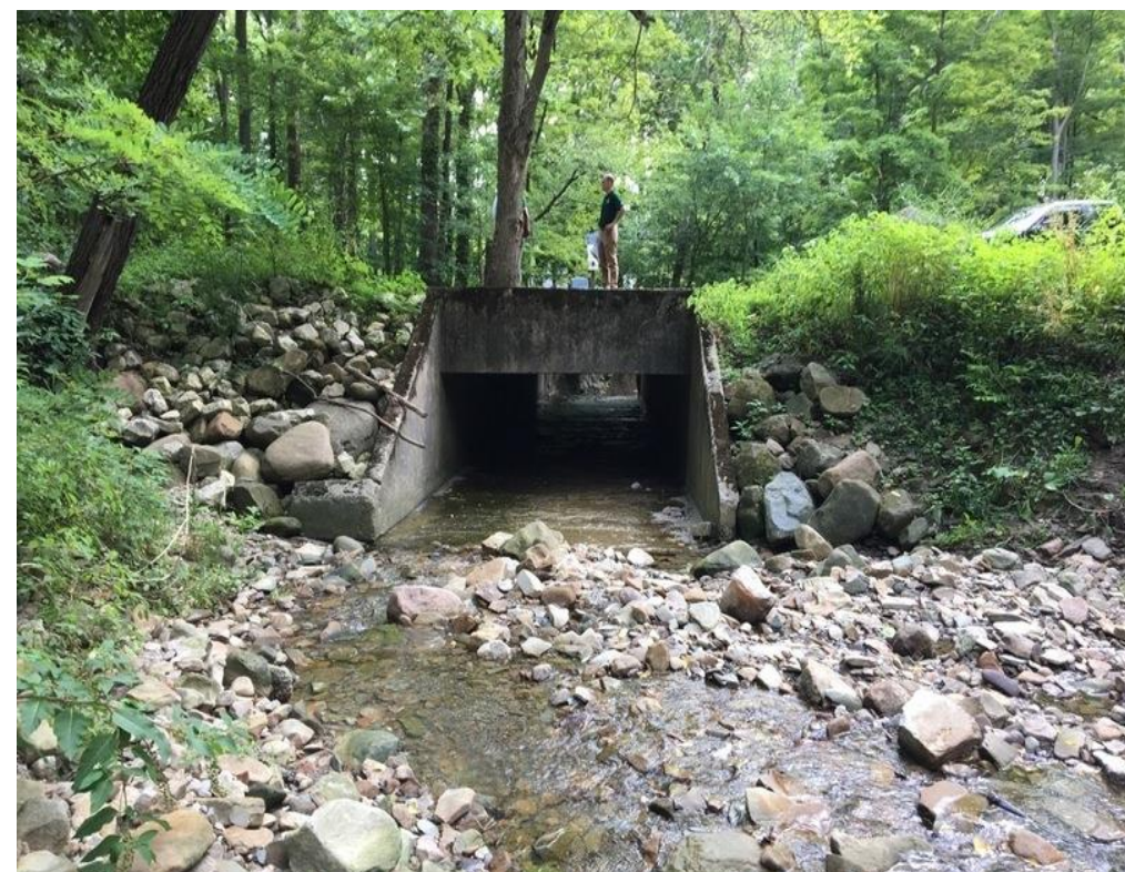
Undersized culvert – Beecher's Brook
